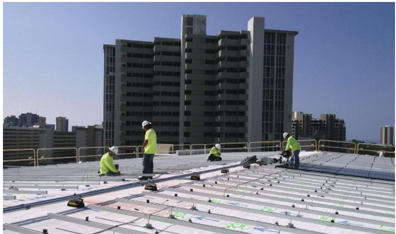
Workers install the hardware used to mount hundreds of solar panels on the gymnasium roof at Hawaiian Mission Academy, which expects its campus to be fully solar powered during the 2013-2014 school year.
